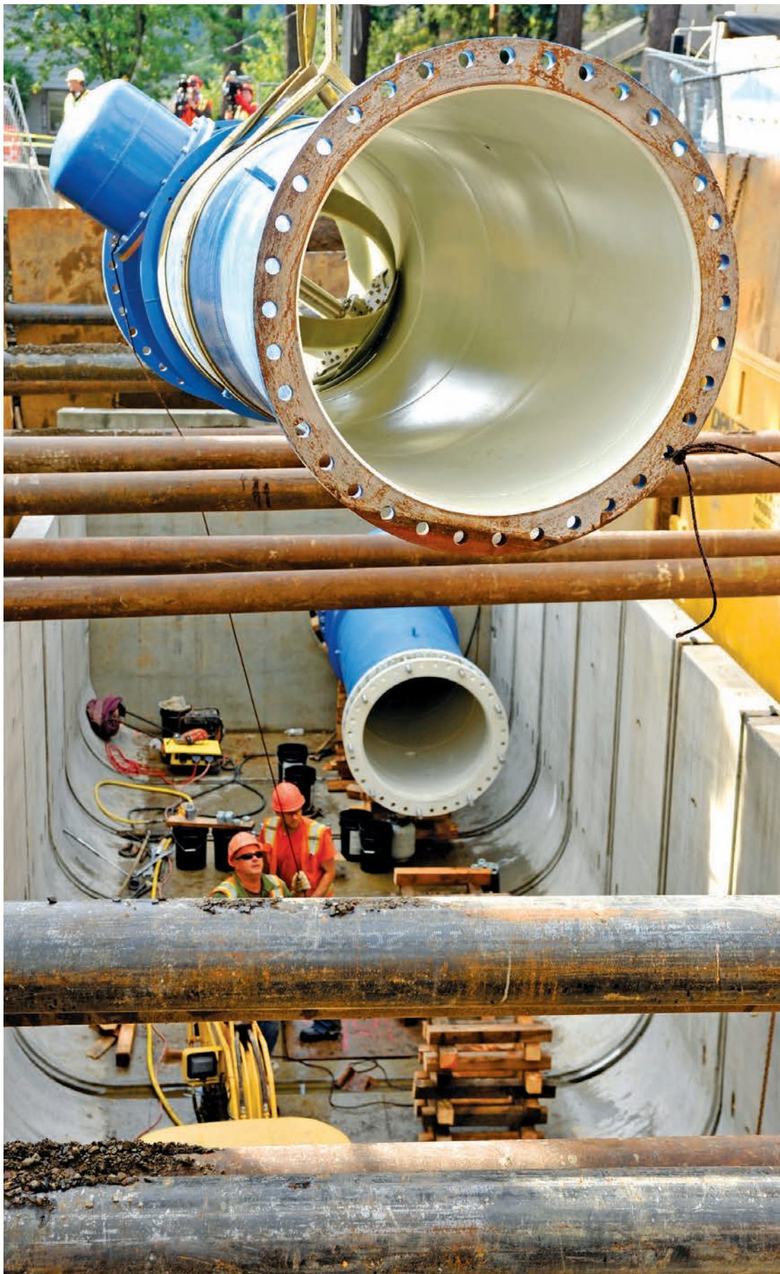
The electrical generating systems were part of a Portland Water Bureau $150 million upgrade. Lucid Energy financed the installation and sells the electricity to the local utility, Portland General Electric. (Photo Sherri Kaven)
