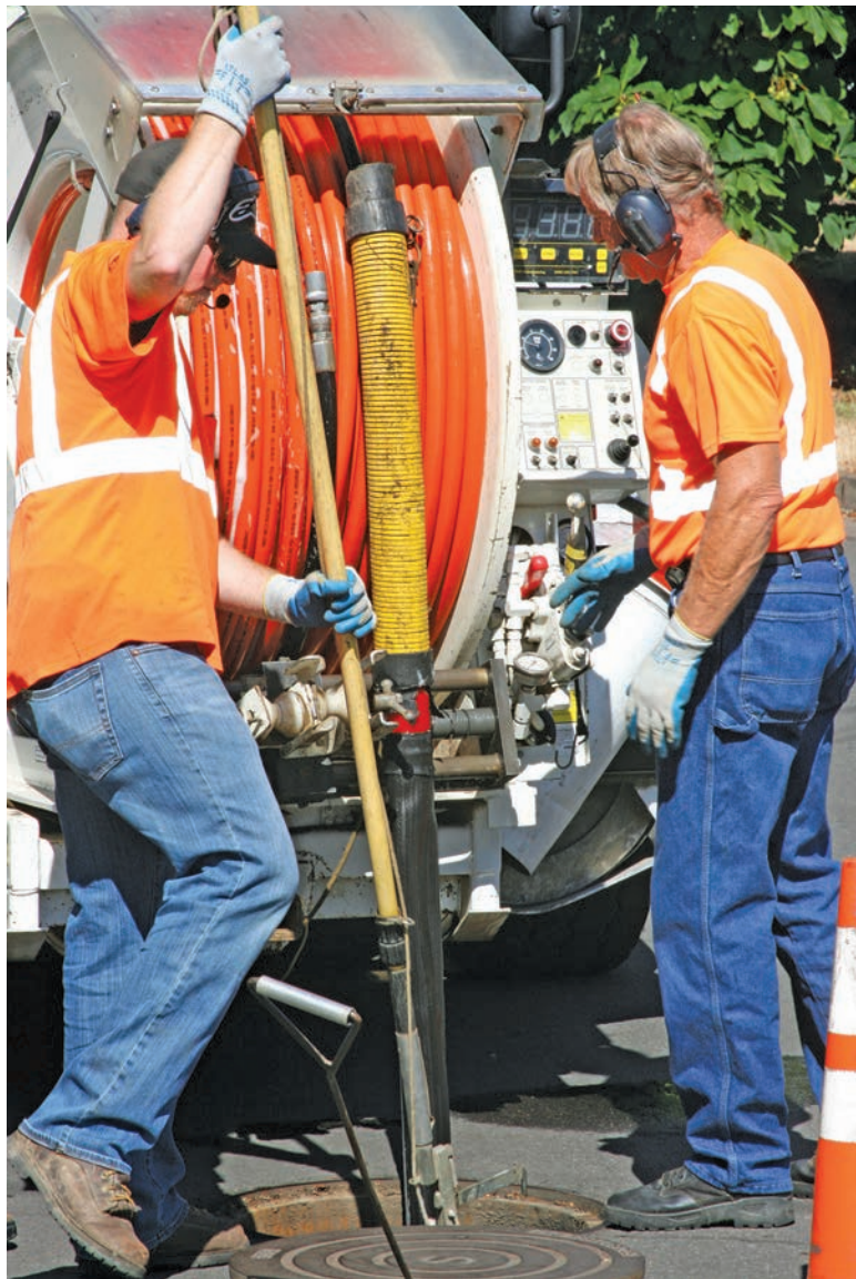
The Ceres crew works in 300-foot runs, from manhole to manhole, when treating its system for roots. Lines are always flushed before the root treatment is applied.
