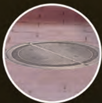
Sewer Force Main Discharge
