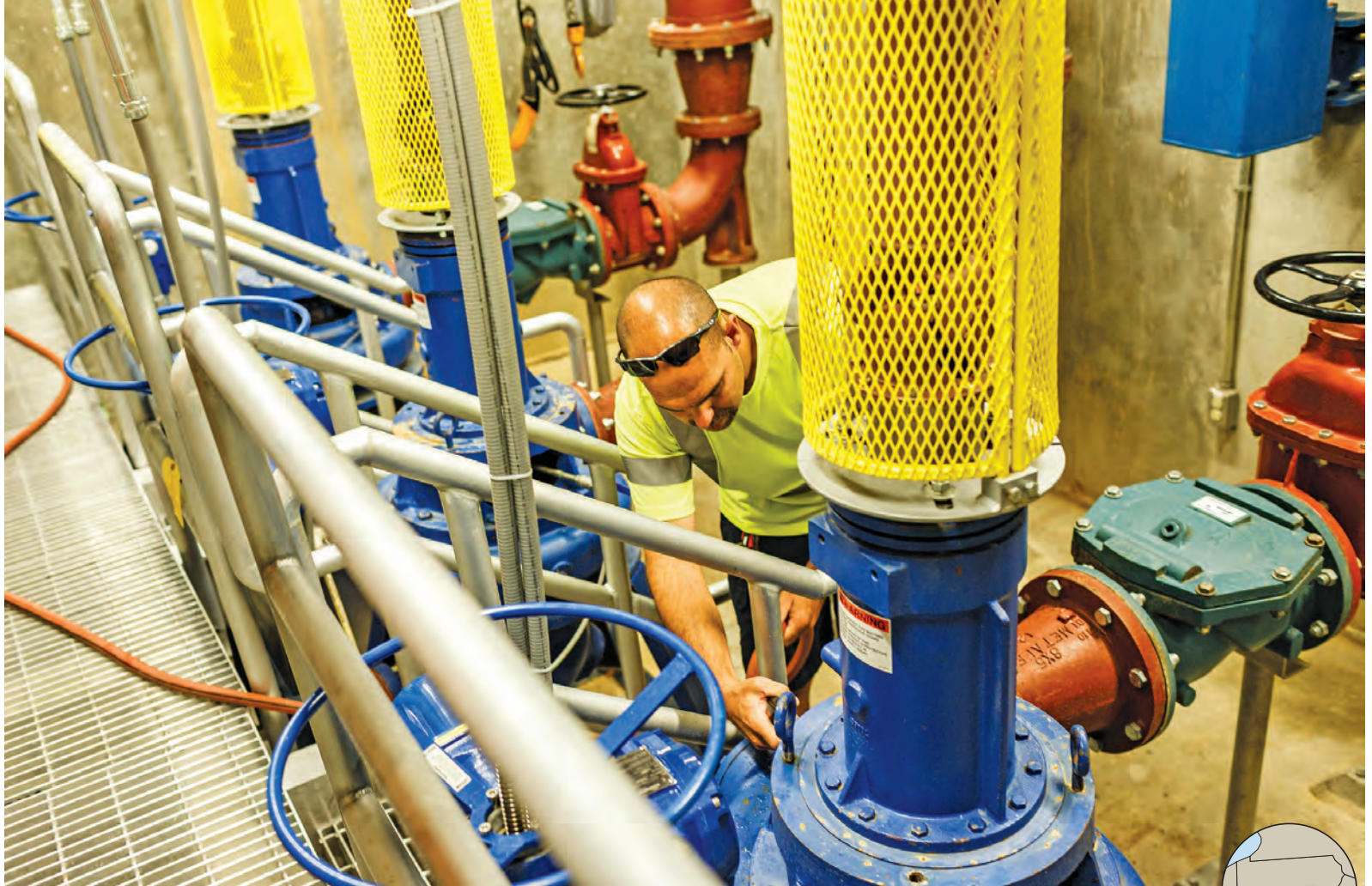
Troy Dehoff checks and cleans pump seals at the Panorama Hills Pump Station, which was built to serve a new commercial and residential development.
