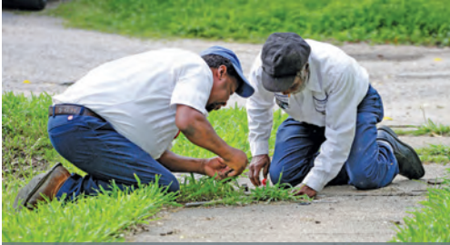
Tallahassee Water Service employees Robert Neal (left) and Charles Fines service a residential water meter.
