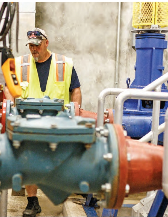
James O'Dell inspects pump station equipment.
