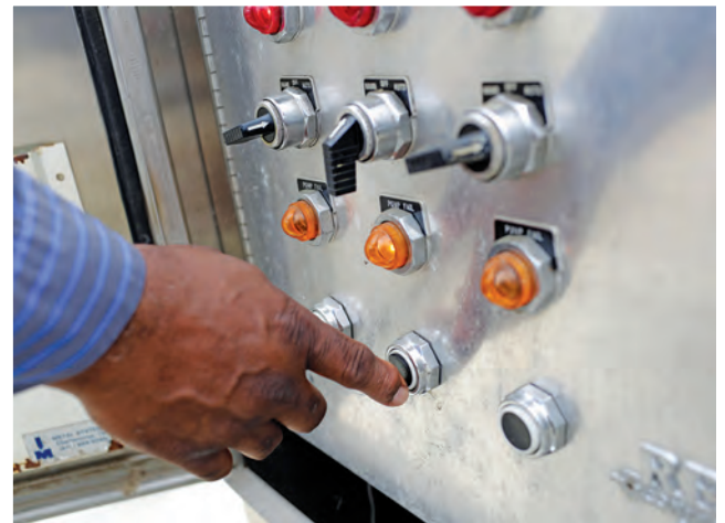
Johnny Robertson checks the control panel at the main lift station.
