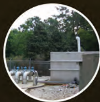
Sewer Wet Wells & Storage Tanks
