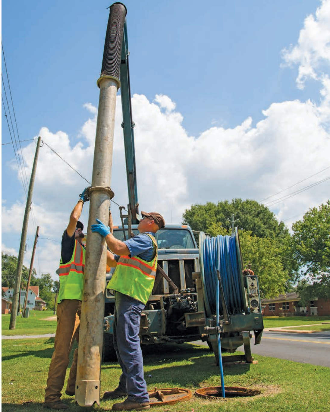
Lynn Gobles (left) and David McAlpin connect extension tubes to the vacuum boom on a Vac-Con jet/vac truck at the start of a sewer cleaning job.
