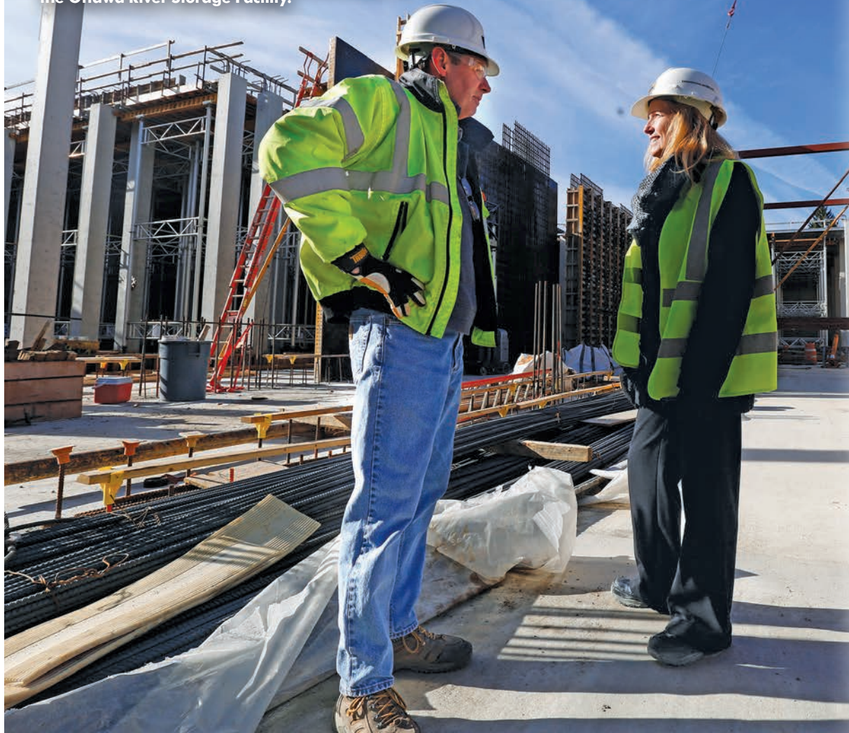
Construction manager Rich McQuade (left) speaks with Julie Cousino, program administrator with the Toledo Waterways Initiative, at the bottom of the Ottawa River Storage Facility.
