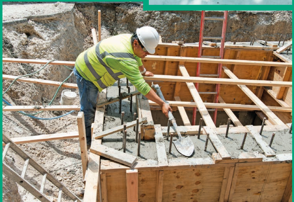
A crew member levels off fresh concrete on the foundation of a new pump station under construction near the Miami-Dade Water and Sewer Department building.
