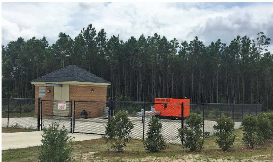
Isle of Wight County's newest lift station — supporting the new Benn's Grant residential development — was outfitted with a Godwin Dri-Prime Backup System (DBS) capable of handling the station's estimated 1,420 gpm flow.
