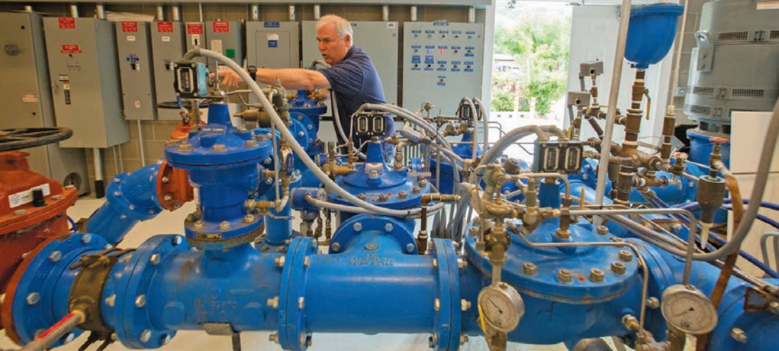
Randy Randall shows how demand charges are saved by using a generator outside the Park Hills Booster Station.
