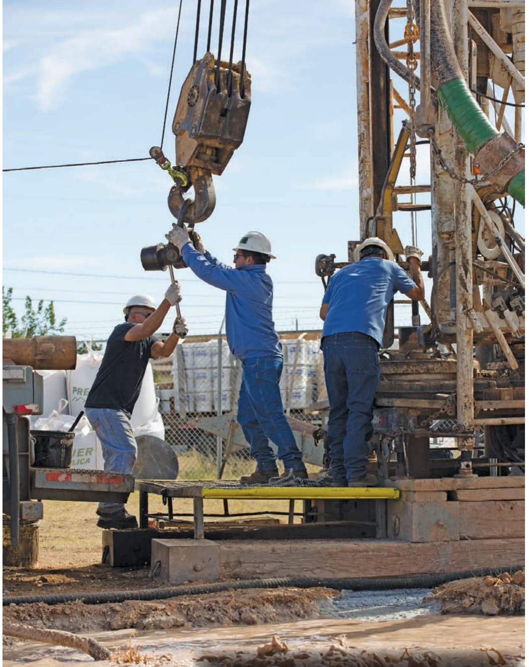
Contractors Mike Flores, Manuel De Haro and Isidro Moreno work on a replacement well for El Paso Water. (Photography by Marcos Fernandez)
