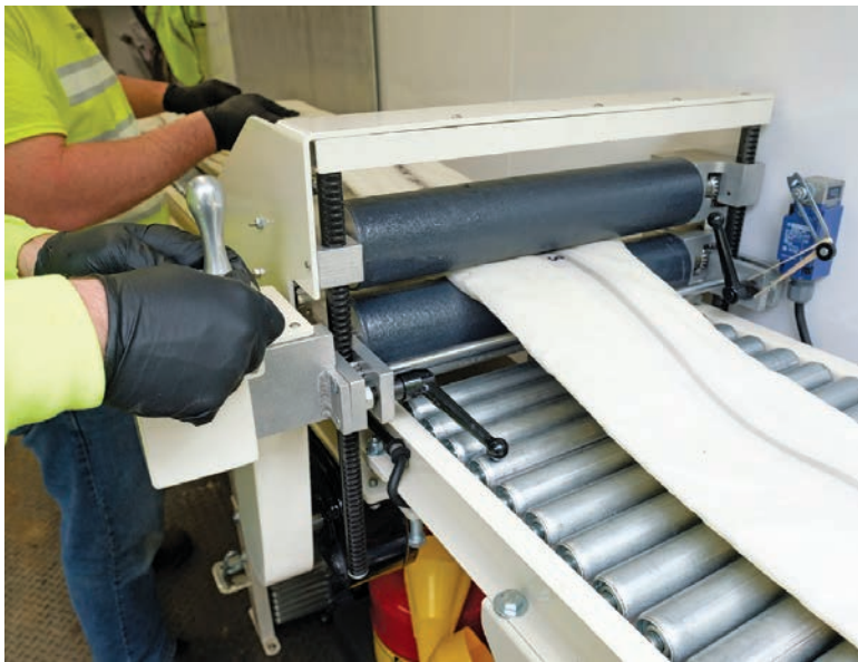
Before installation, liners must be impregnated or “wetted” with a catalyzed resin. In some cases, prewetted liners are sent to the job site in a sealed container, but the wetting process can also take place on the job site in a purpose-built truck or trailer.
