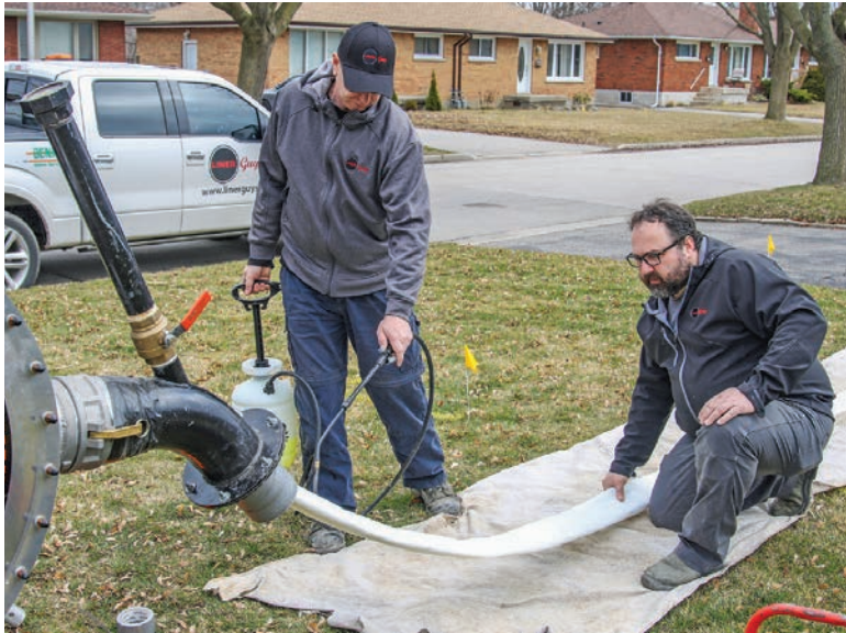
A fresh liner is lubricated and fed into an inversion unit for installation in a 4-inch-diameter sewer lateral.
