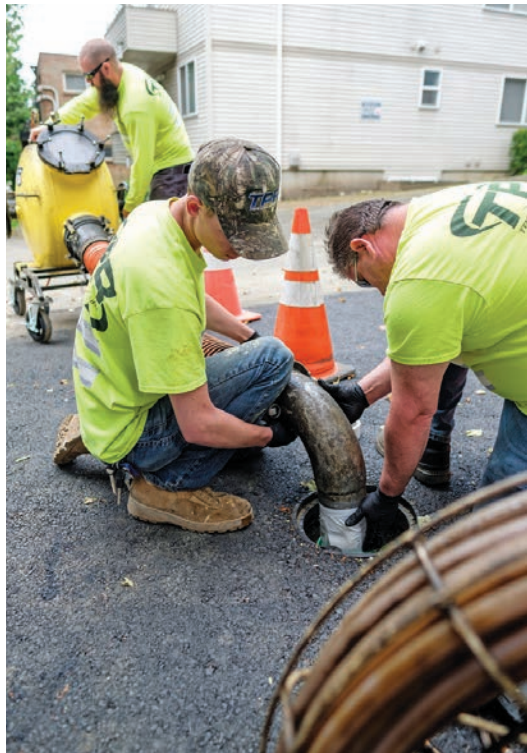
A crew shoots a liner into a residential sewer lateral from a cleanout in the driveway.
