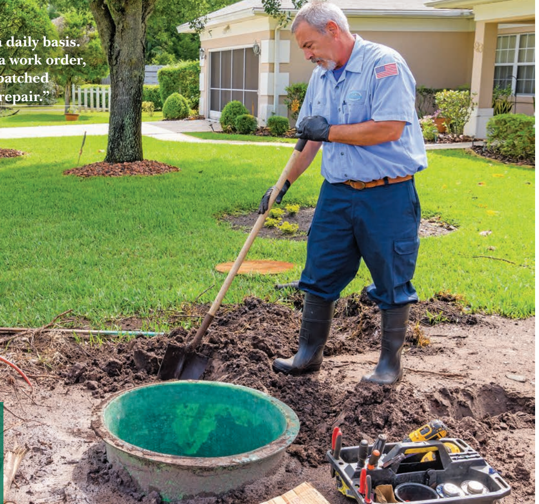
Utility Foreman Bryan Parreso (left) and technician Don Abbott work on a Pretreatment Effluent Pumping tank installation at a new home site in Palm Coast.
