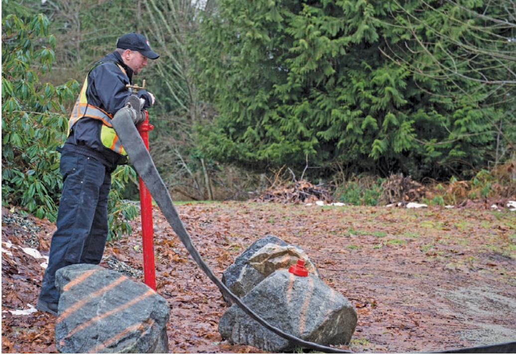
Tyler Musgrove connects a hose for routine pump flushing. Town water is pumped from three wells and two reservoirs.
