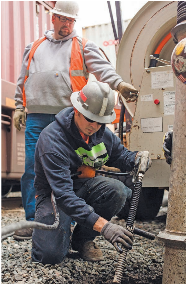
Hydroexcavation safety takes planning and teamwork. Having a second person on site to watch the operator and keep an eye on everything is critical. (Photography by David Ryder)
