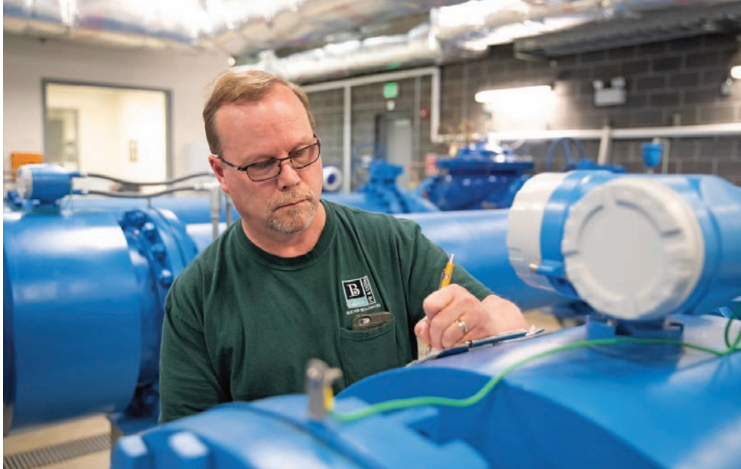
Senior operator Harry Repine checks flow meter readings on 24-inch pipes at Bremerton’s Advanced Disinfection Facility.
