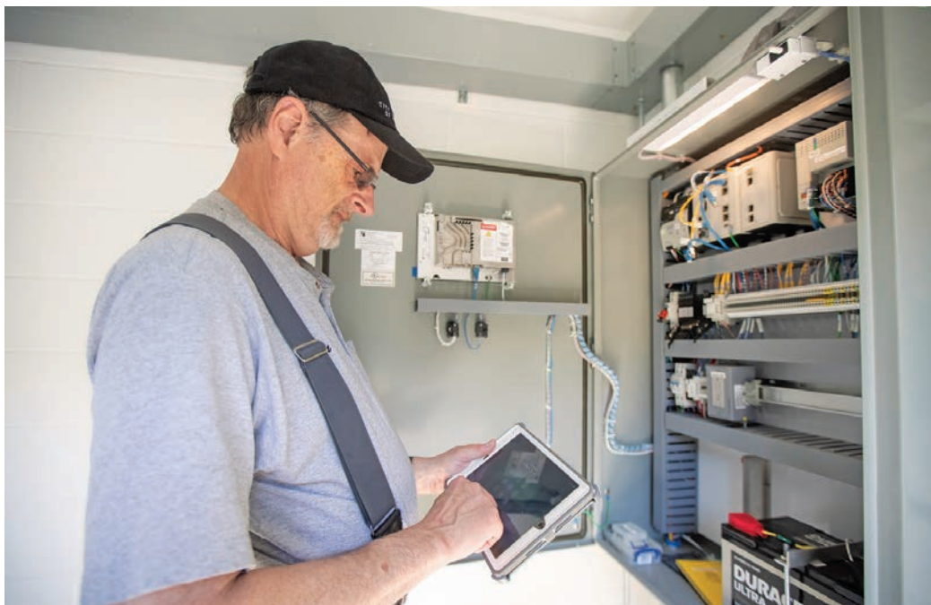
Utility instrumentation and control specialist Tom Baker cleans a fiber optic cable in a utility room next to the Casad Dam.
