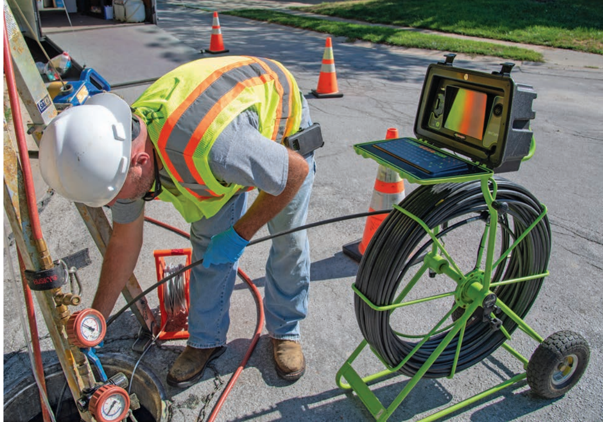
Sean Kelley uses an Envirosight VeriSight Pro camera to inspect a spot liner after installation.
