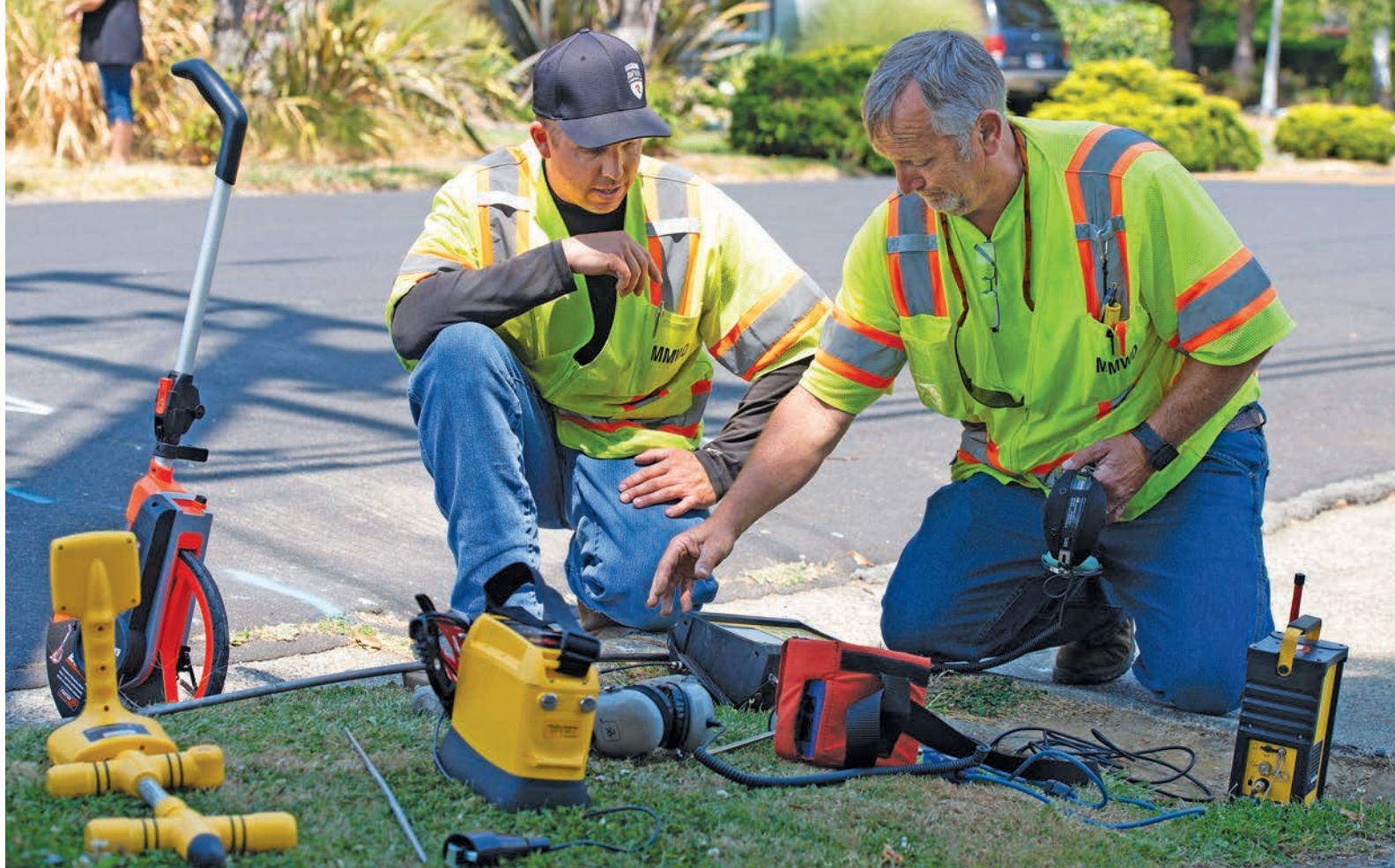
Left: Utility systems specialist Kevin Barkdull, a member of the Marin Municipal Water District's Leak Detection Team, uses a ground mic to listen for leaks in a waterline. Above: Barkdull and water systems technician Jesse Obrochta set up SubSurface leak detection equipment. (Photography by Lezlie Sterling)
