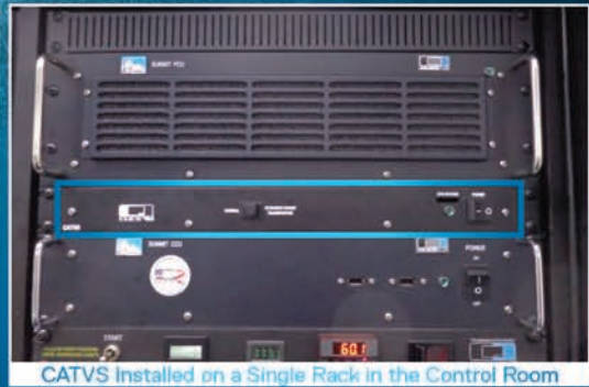
CATVS Installed on a Single Rack in the Control Room
