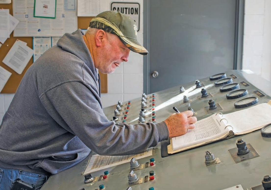
Water Treatment Manager Randy White back-washes the flocculation basin for routine cleaning.
