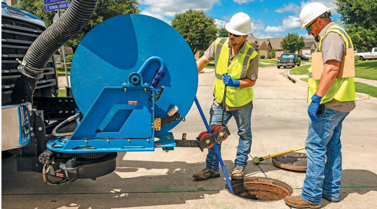
Bryce Skotnicki (left) and Leston Dhane clean a sewer main using a PipeHunter combination truck.
