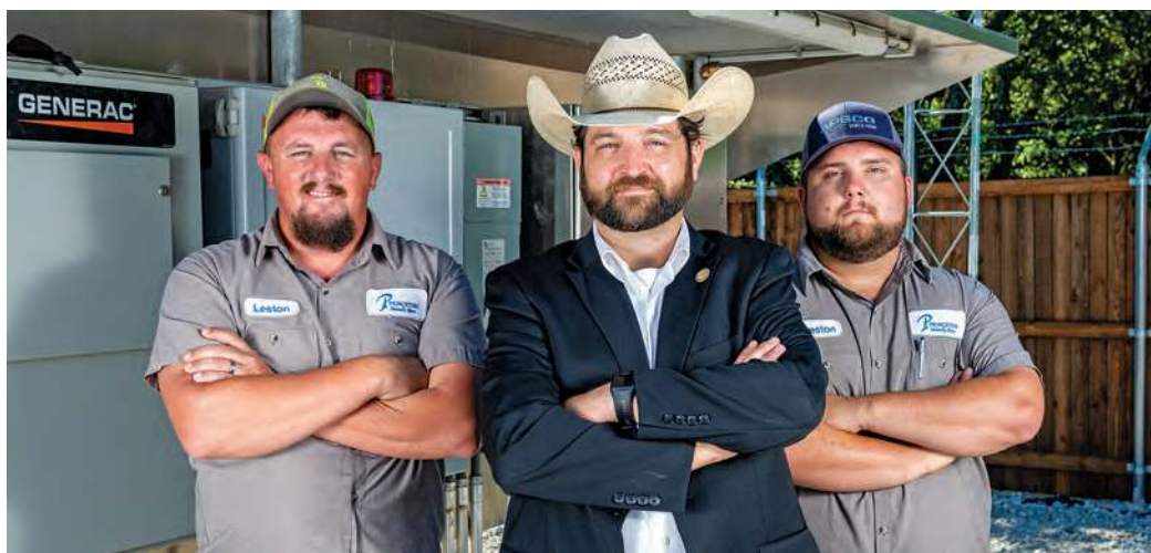
The Princeton wastewater crew includes (from left) crew lead Leston Dhane, Director of Public Works Tommy Mapp and Public Works Superintendent Preston Jones.
