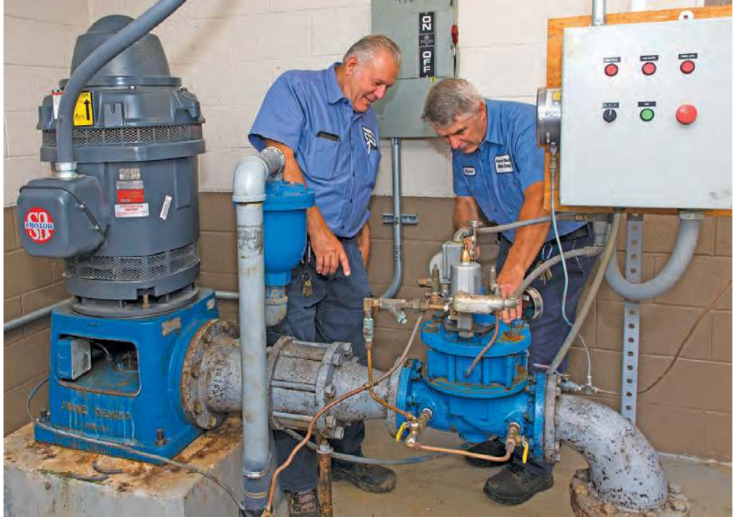
Superintendent Wayne Bugay (left) and Mike Perzanowski check the operation of Elton Well 2A, consisting of a US Motors and Crane Pump system. This is the utility's largest well, producing approximately 350 gpm.
