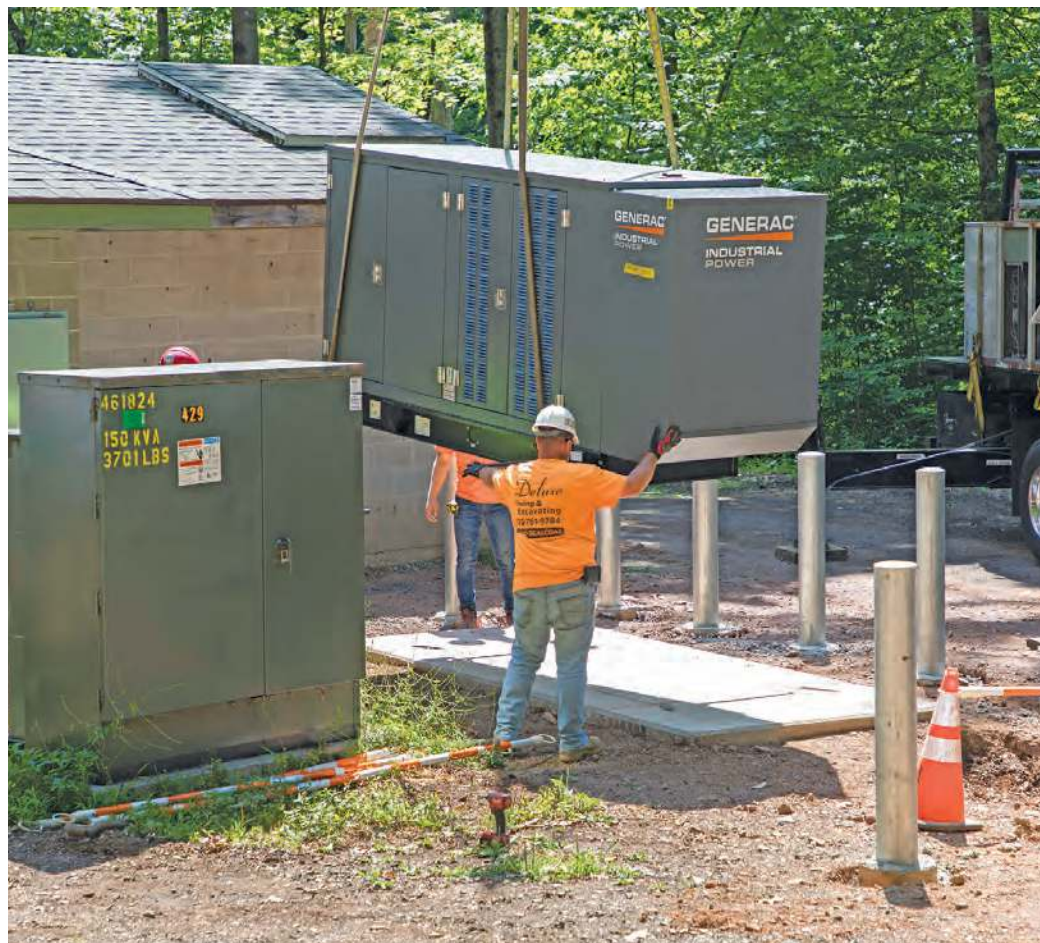
A new Generac generator is placed on its pad at the Elton Road wellfield, assuring continued operation during power losses.
