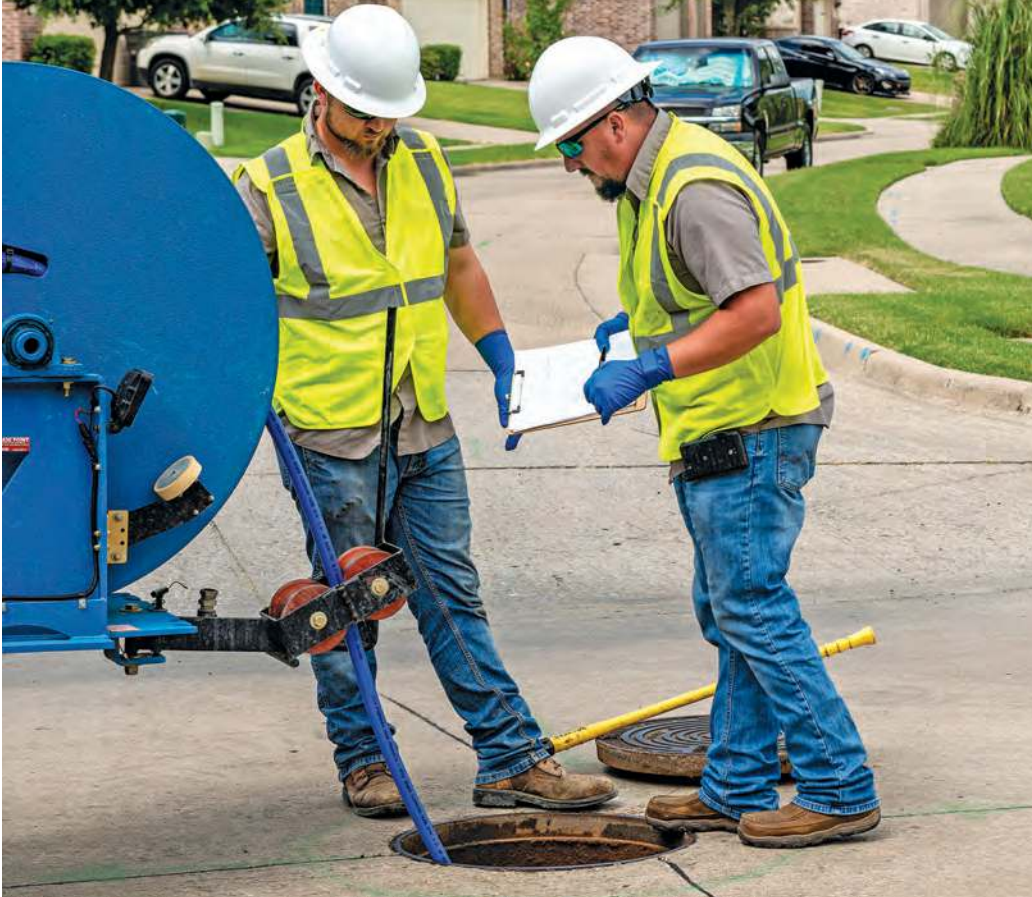
Wastewater technician Bryce Skotnicki (left) and crew lead Leston Dhane log the condition and cleanliness of a sewer main prior to cleaning. This is the department’s policy every time a manhole cover is opened.
