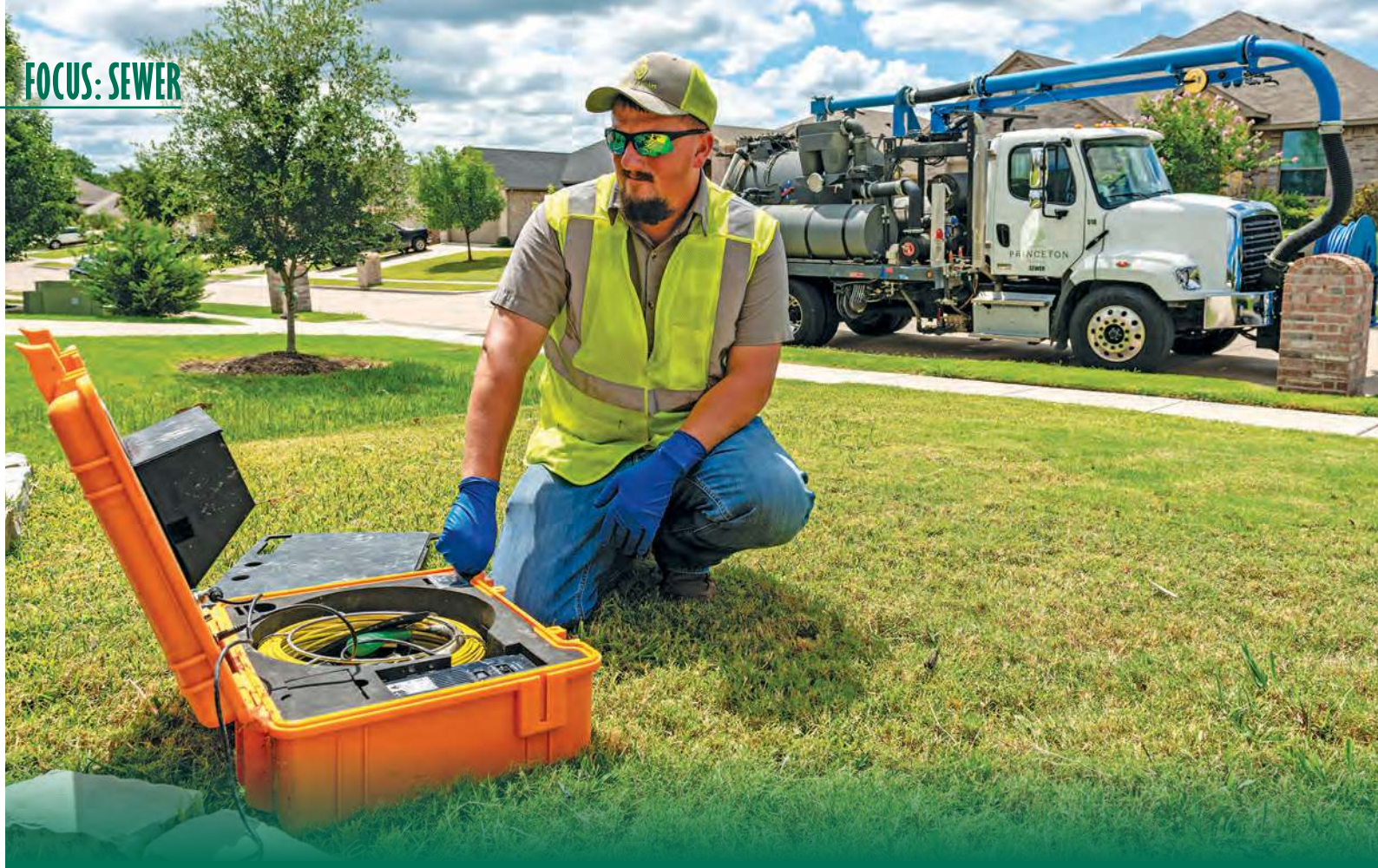
Princeton (Texas) wastewater crew lead Leston Dhane watches the monitor on a PipeHunter inspection camera during a residential sewer lateral inspection. The department offers this service free to Princeton residents. (Photography by Olivia Ogren-Hrejsa)
