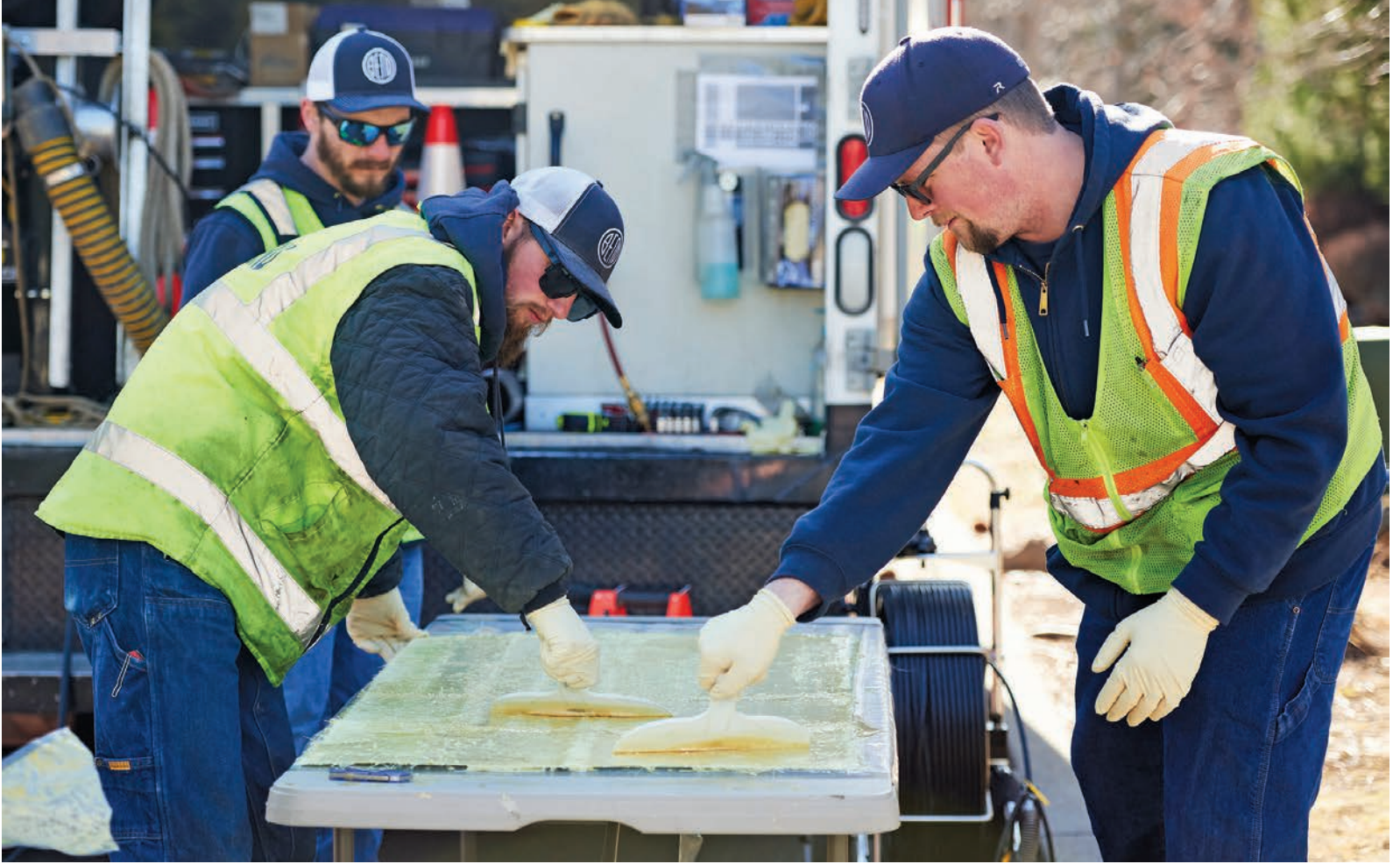
Bend Collections Utility workers Brent Suing (left) and Joe Johnson apply two-part resin to a fiberglass patch for a sewer line repair.
