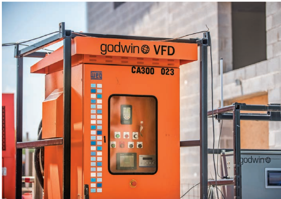
Pumps were fitted with Godwin variable frequency drives, enabling operators to control the motor speed and ensure optimum operating efficiency throughout the project.
