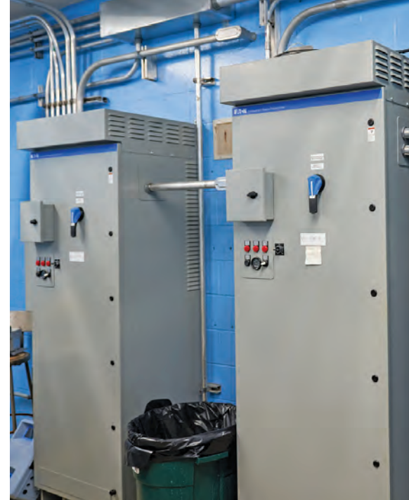
Groton also installed a new Eaton Freedom 2100 Motor Control Center in the Whitney Pond Wells pump station.
