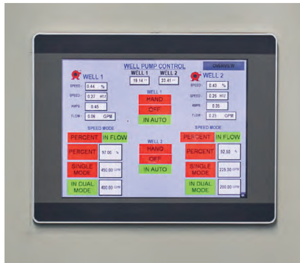
The new SCADA control panel at the Whitney Pond Wells pump station gathers information in real time and sends it to the Baddacook facility.
