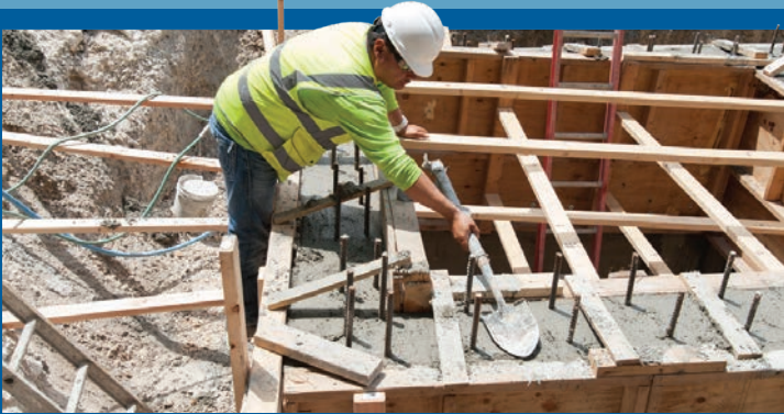
A crew member levels off fresh concrete on the foundation of a new pump station under construction near the Miami-Dade Water and Sewer Department building.
