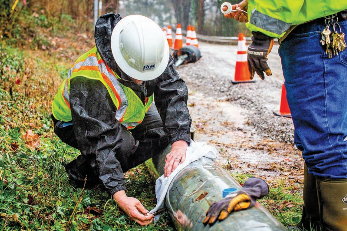
First Utility District Operations Manager Brad Brummett assists Knox County in setting up temporary pumps after Bluegrass Lake overflowed, causing flooding of surrounding neighborhoods. Knox County asked First Utility District to advise as well as offer technical expertise.
