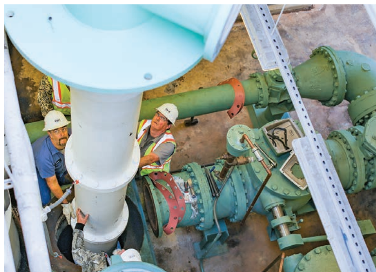
Top: Davin Olafson, Scott Harrison and Rodney Lawson (from left) install replacement pumps at the Ten Mile Pump Station after the February 2019 flood destroyed them.
