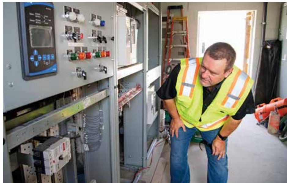
Burris checks over the new electrical control building's MCC units prior to energizing the building.
