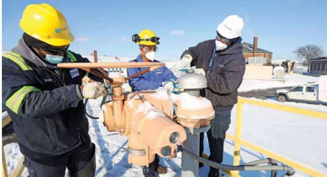
Maintenance technicians Marcus Jackson (left) and Hawun Howard (center) service pump station gate operators with team lead Lorraine Lewis.
