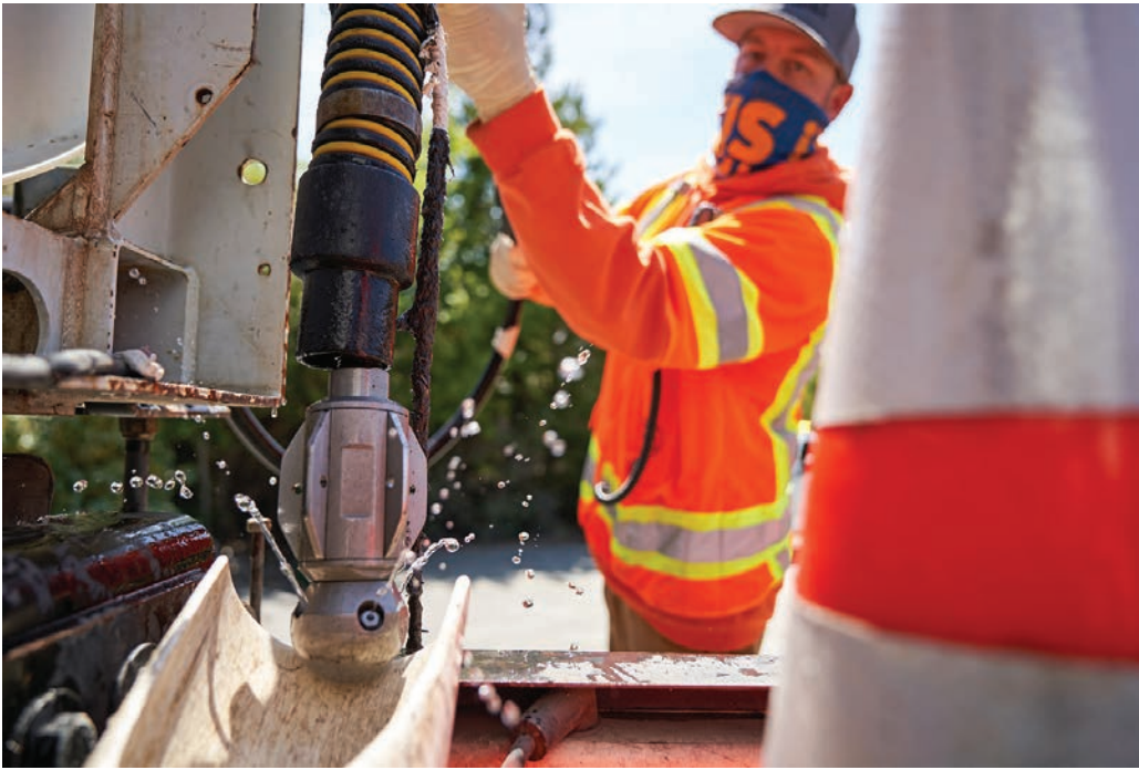
Collections worker Darrell Proschold rewinds the jetter hose after completing the last of several routine cleaning runs in a residential area north of San Francisco.
