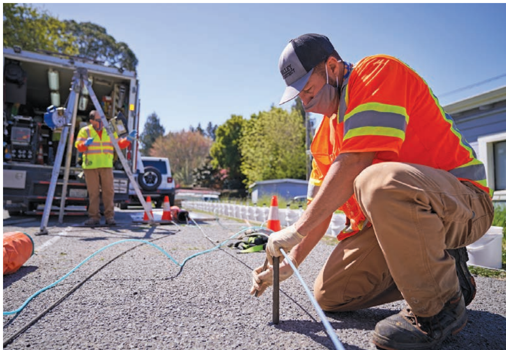
Ross Valley Sanitary District collections worker Ricky Smith prepares the inflation line for an epoxy patch carrier. Ross Valley is one of California's oldest wastewater utilities, with aging clay pipes that require regular maintenance and repair.
