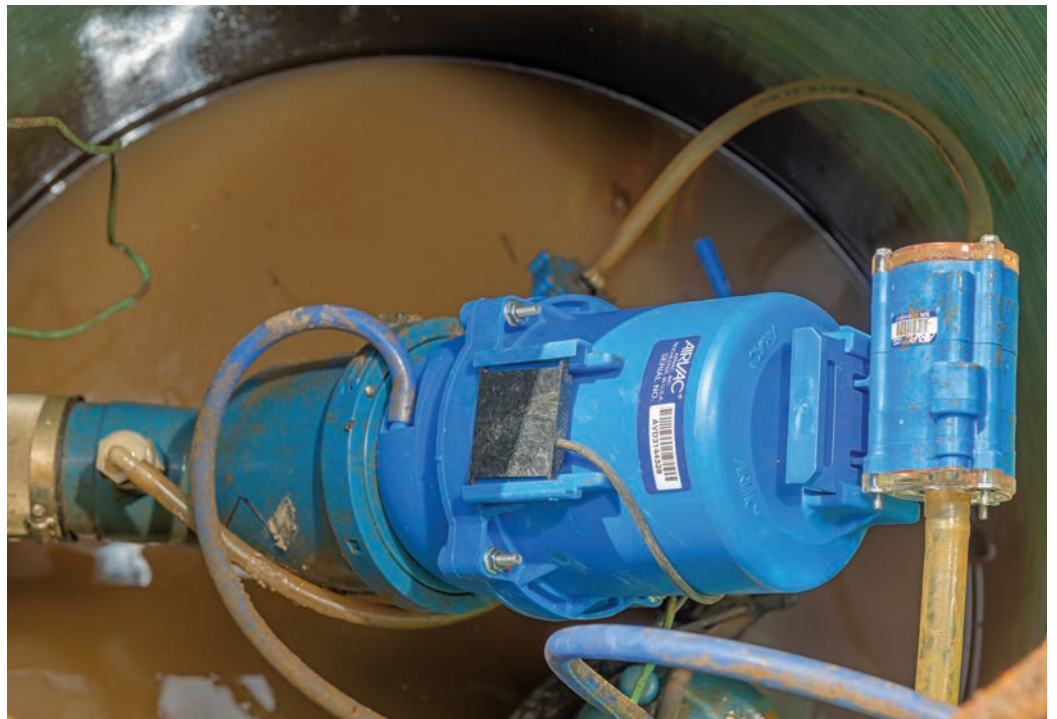
The newly installed valve body and sensor in one of the district's 372 pit connections.
