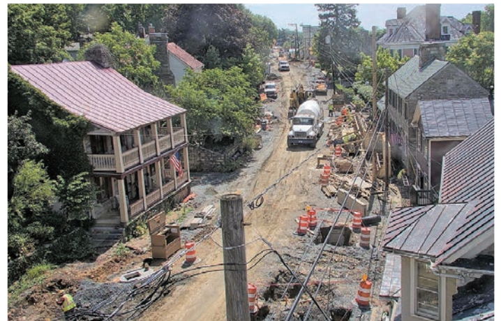
The core of the project included new water, sewer and stormwater systems, a complete rebuild of Route 9, burial of all aerial utility lines and new conduit for fiber optic lines.
