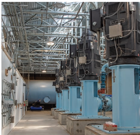
At the heart of the EL 47.5 project is the 12,800-square-foot pump station, which will reduce groundwater depletion by up to 73 million gallons per day.
