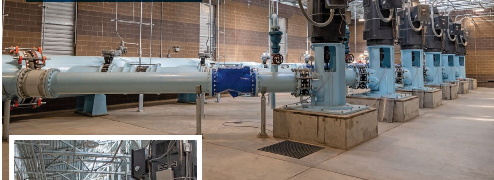
The first pump distribution system in the Odessa Ground Water Replacement Project, called EL 47.5, includes nearly 9 miles of pipe, six pumps and a pump house.
