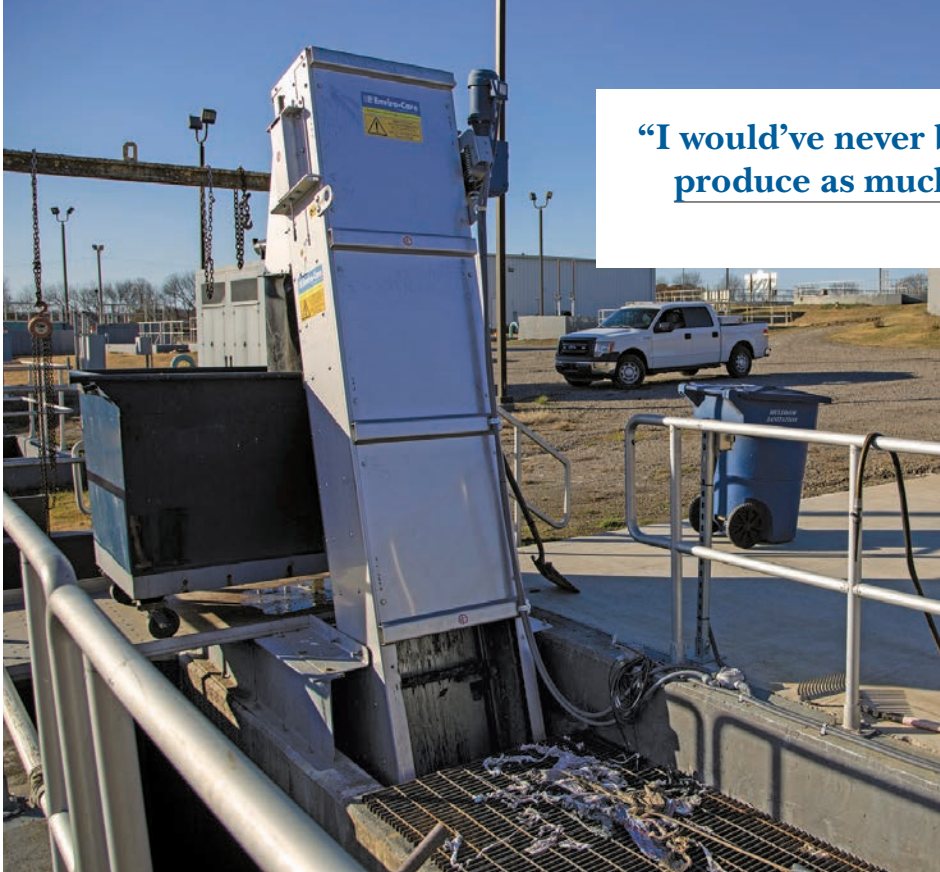
The Enviro-Care bar screen machine at the wastewater treatment facility in Muldrow.
