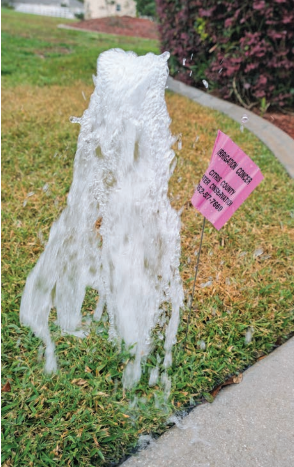
A broken or missing sprinkler head not only wastes a tremendous amount of water, it can also cause serious damage to a homeowner’s landscaping. Problems like this are flagged by the water conservation specialists and brought to the homeowner’s attention.
