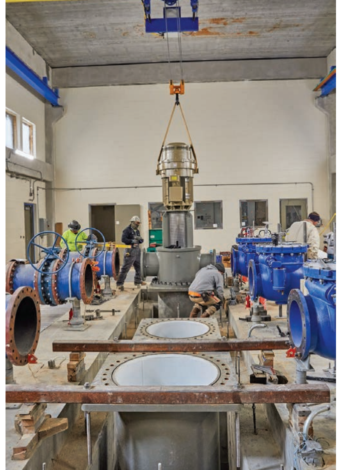
Workers install a vertical turbine at the Macon Water Authority’s new booster facility.
