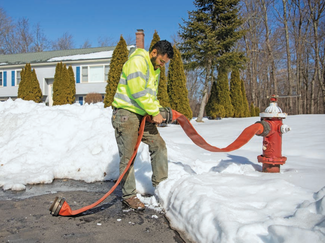
Jonathan Gonzalez-Rosario attaches a hose to a fire hydrant before flushing a segment of the water system.
