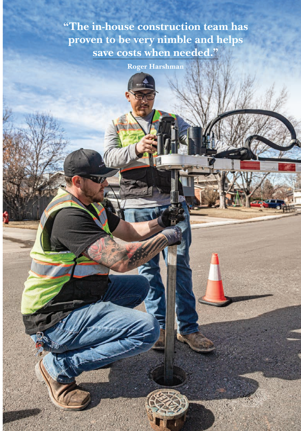
Utilities operators Nick Craig (left) and Trueman Sanchez exercise a water main valve with a Wachs Valve Maintenance System.
