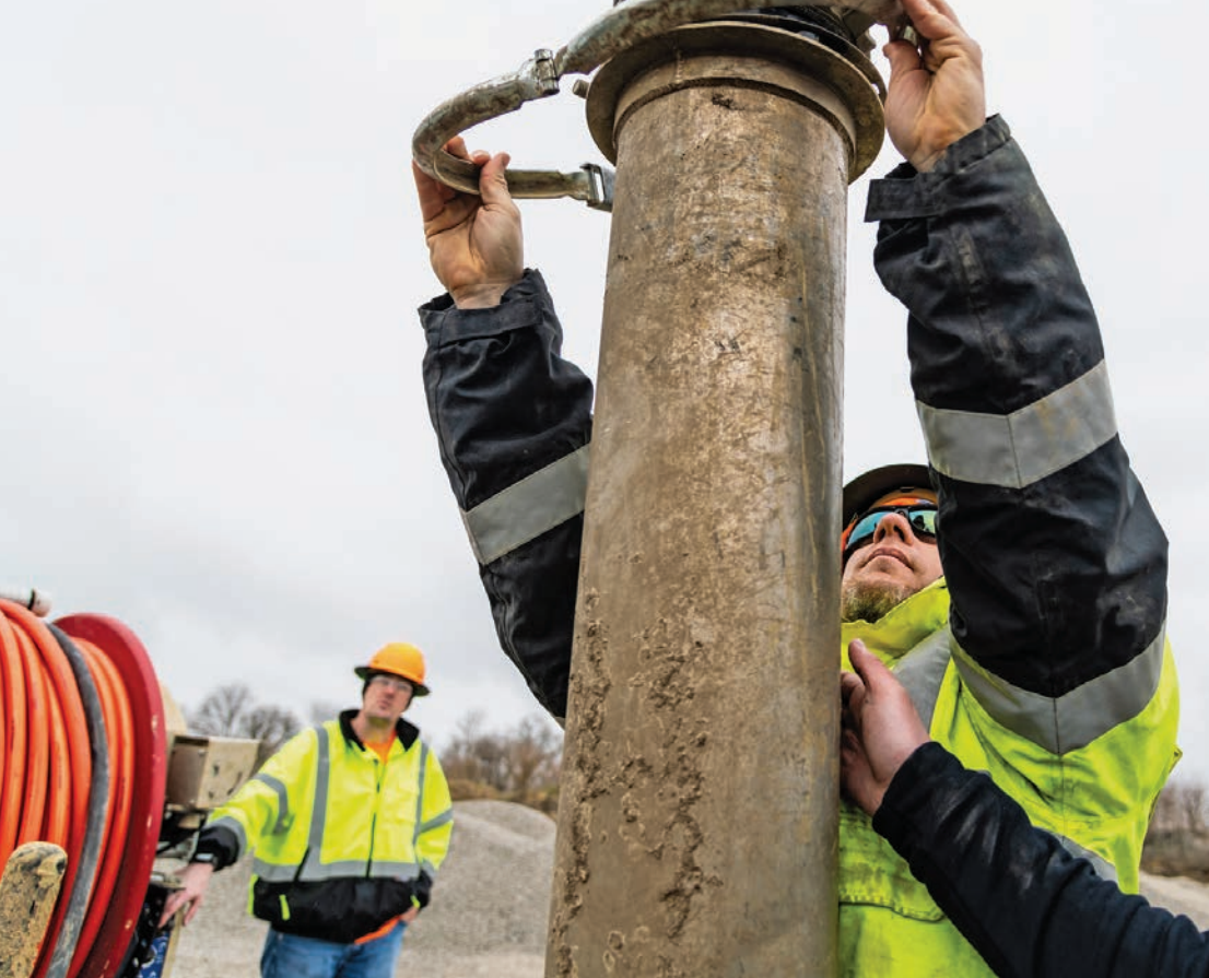
Aaron McLaughlin sets up to hydroexcavate for the installation of a fire hydrant.
