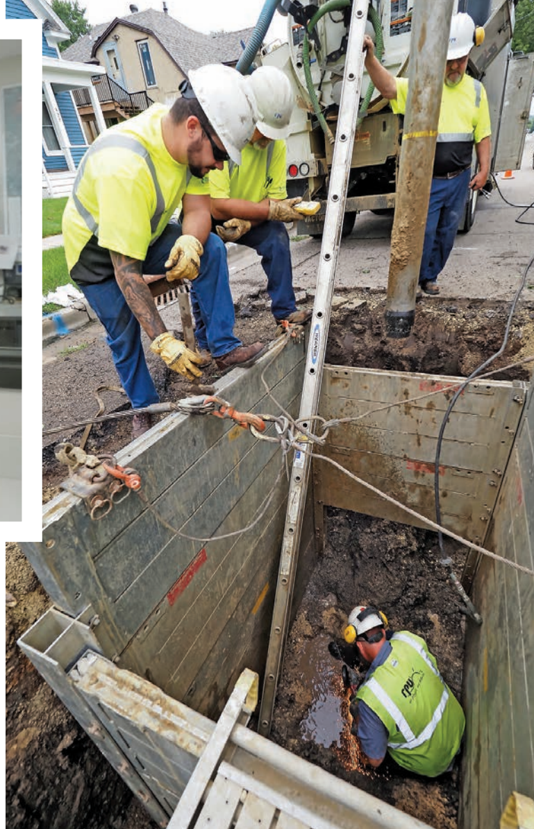
Putzier prepares a water line for a new gate valve. Above from left are fellow lead distribution workers Blee, Quandt and Rich Rain.
