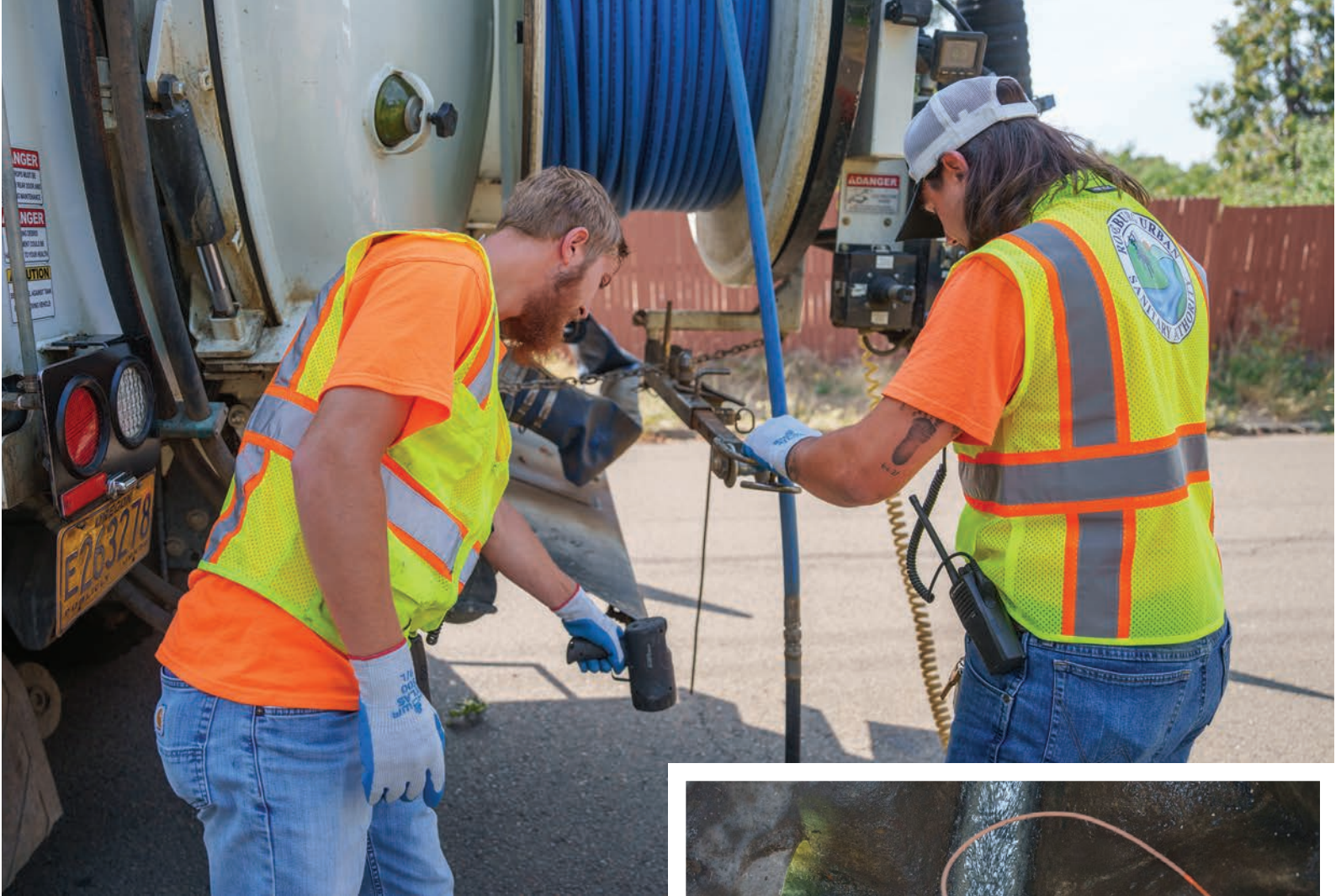
Roseburg Urban Sanitary Authority crew members Nic Soule and Devin Freeman flush a sanitary sewer main prior to inspection.
