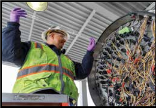
Ray Camacho replaces UV lamps for the Groundwater Replenishment System's Trojan UV Phox UV reactor core.
