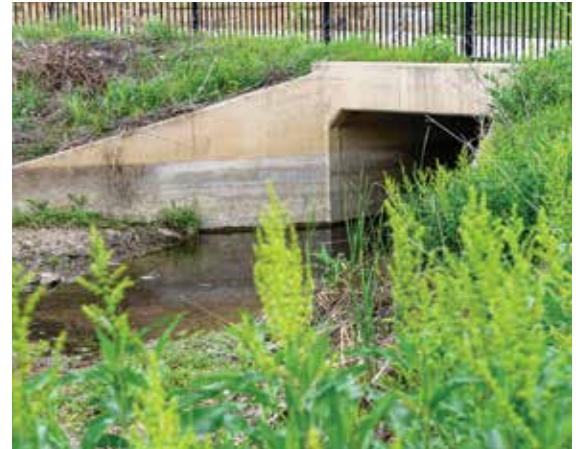
Clear visual evidence of the decreased water level is recorded on the concrete foundation of a bridge at the Cottonwood Creek Trail.
