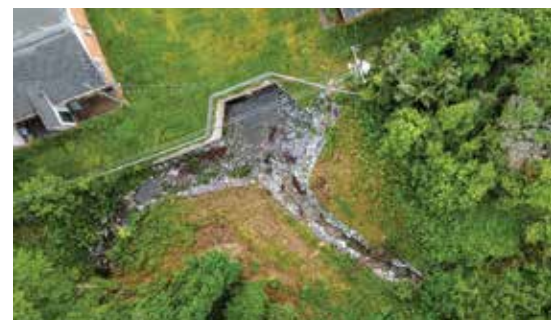
A double-barrel box culvert safely guides rainwater runoff under the housing development at the Cedars East Storm Drainage Improvement Project in Charlotte, North Carolina. The project wrapped up in 2021 and has eliminated flooding issues from creek runoff. (Photography by Logan Cyrus)
