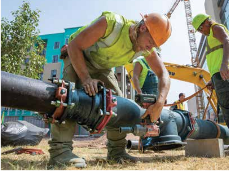
Contractors Justin Gorter (left) and Johnny Gorter tighten retainer gland bolts on a water line connected to the Sixth Street Project.
