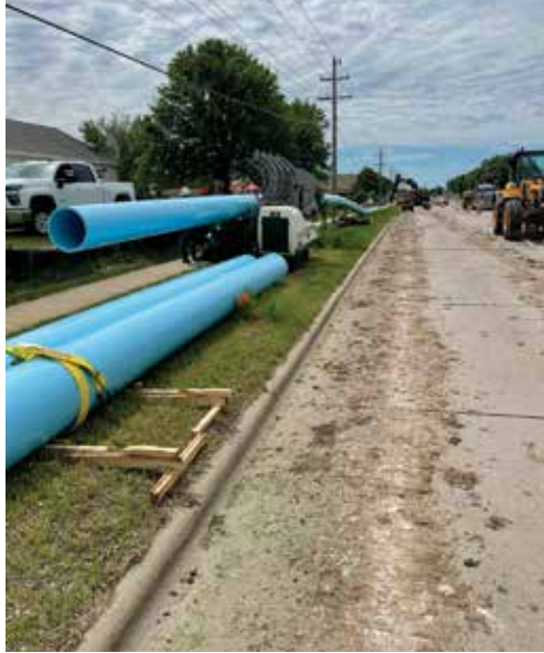
The Siteworks crew replaced the existing mains with 16- and 20-inch fusible PVC.
