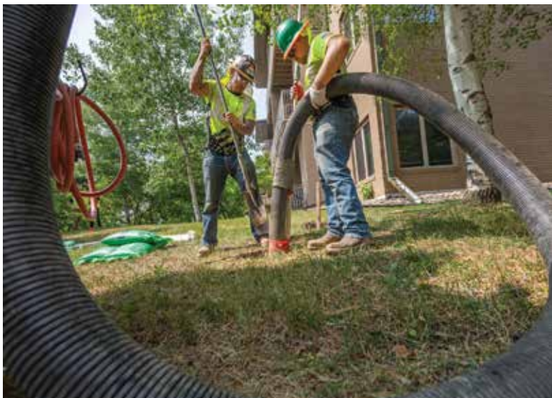
Izzy Salas (left) and Thomas Greene expose a water line for the cathodic protection retrofit project in Sioux Falls.
