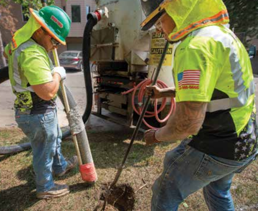
Thomas Greene (left) and Izzy Salas use a vacuum excavator to expose utility lines.
