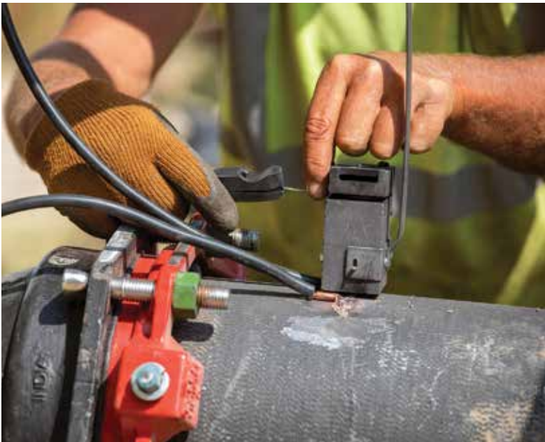
A contractor installs cathodic protection on a new ductile iron water main.
