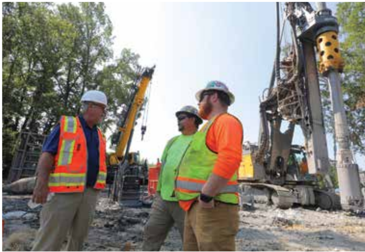
Monty Ledbetter (left) talks with the crew near the Lake Hamilton crossing site for the 17-mile gravity line that will feed Hot Springs' new water treatment facility.
