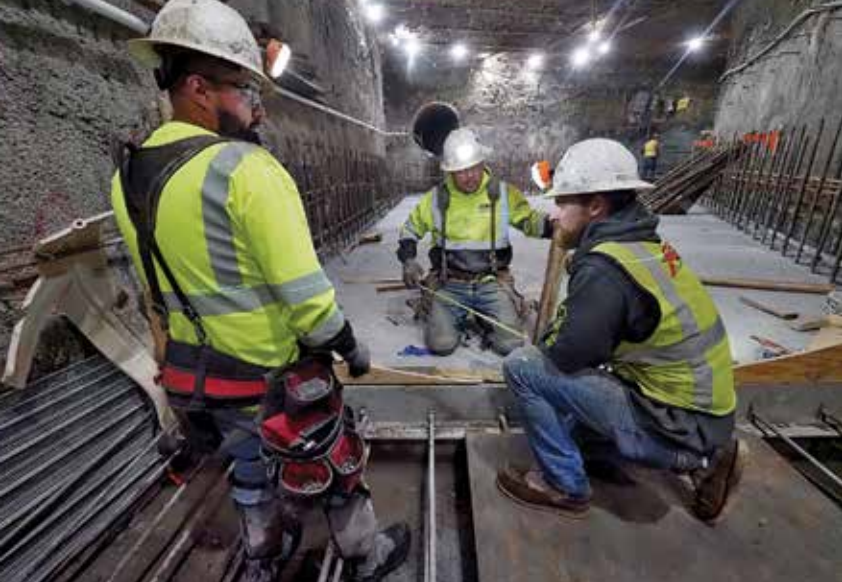
PCI Roads workers Rigo Munoz, Cesar Beceria and Connor Vtschinski (from left) check measurements and alignment as construction progresses in the tunnel.
