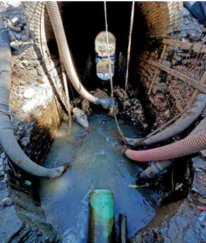
Remnants of the original 1883 storm sewer outlet frame a network of hoses working to clear a settling basin where the tunnel nears its end at the Mississippi River.
