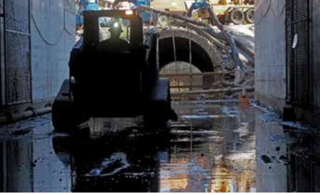
A PCI Roads worker drives a skid-steer through the last segment of the tunnel.
