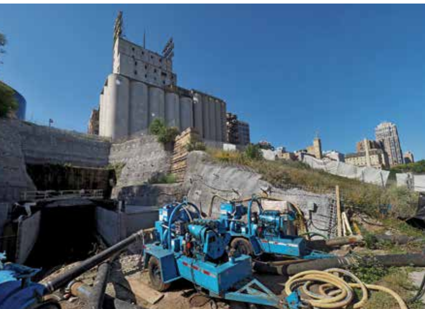
A cluster of pumps and hoses work to drain a settling basin where the tunnel project nears its end at the Mississippi River, with the city's old mill district in the background.
