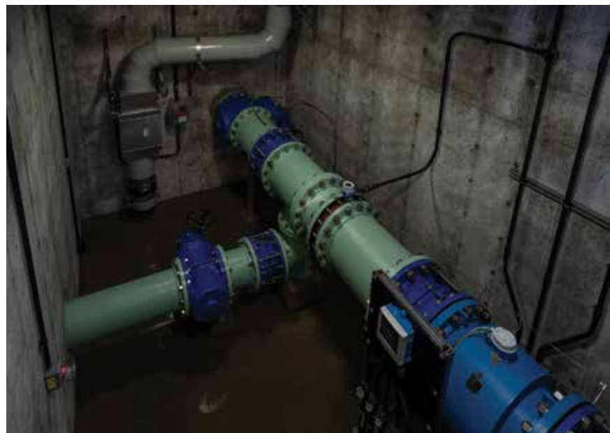
The construction of Lift Station A included four submersible pumps located in a dual-chamber, cast-in-place concrete wet well.
