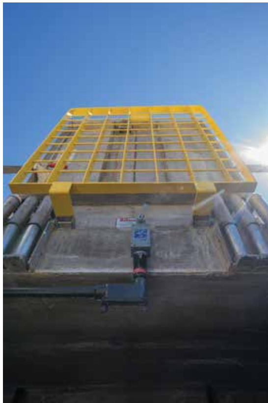
Fourteen BILCO doors provide safe access to pumps, process pipes and grinders for routine service and maintenance.
