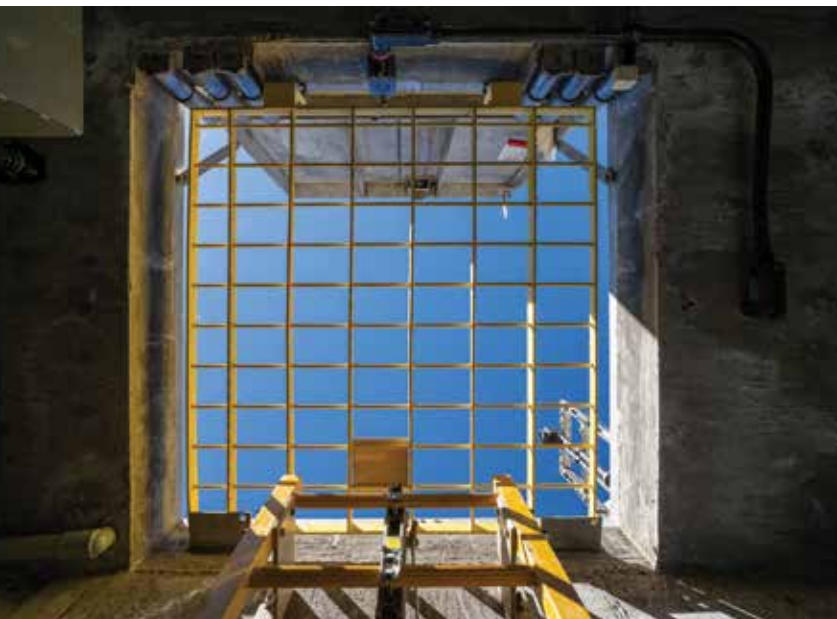
One of the biggest challenges for the Northglenn project was a 54-foot vertical excavation for the wet well on a very tight geographical footprint.
