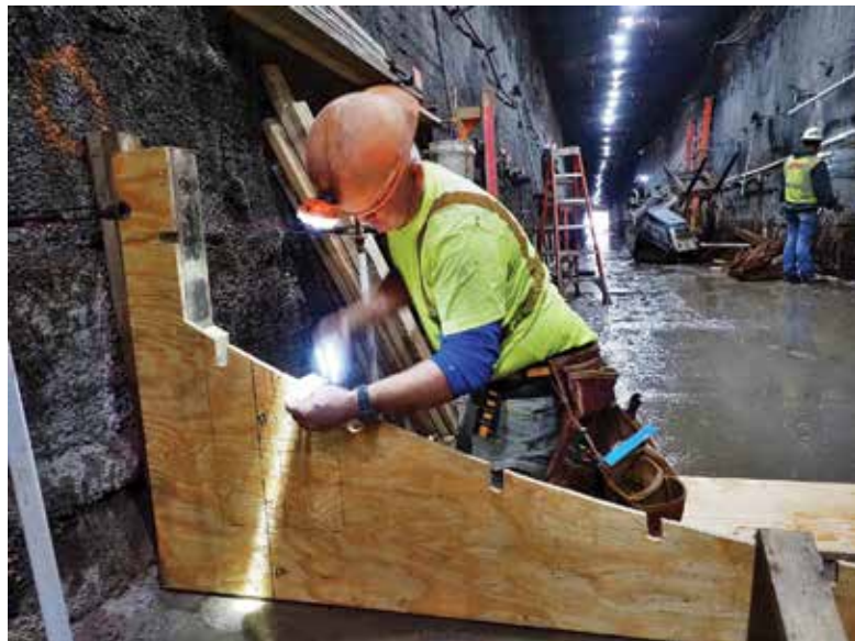
PCI Roads worker Chad Alleckson builds concrete forms for the floor of the Central City Parallel Tunnel Project.
