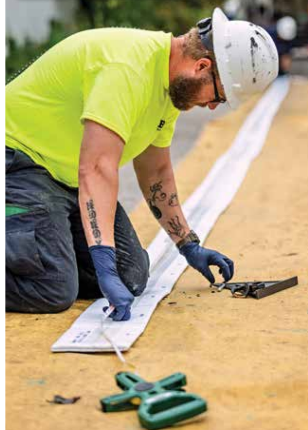
Matt Wagner from BLD Services measures a long section of felt tubing as they prepare to line a sewer lateral at a Columbus residence.
