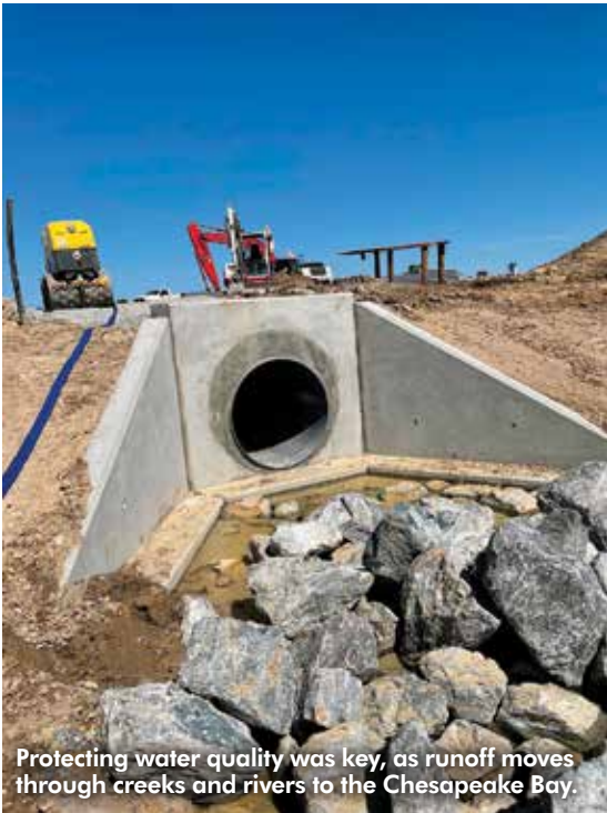
Pipe was installed in trenches from 3 to 7 feet deep, with cover ranging from 2 to 4 feet.
